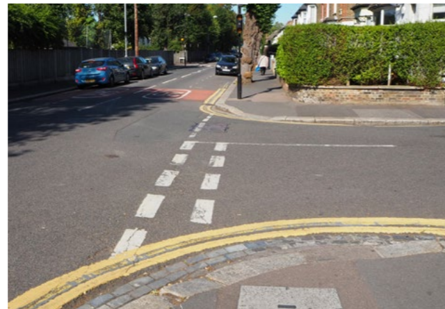
Dropped kerbs with an upstand of more than 6mm can create a barrier for people using a walking aid.
